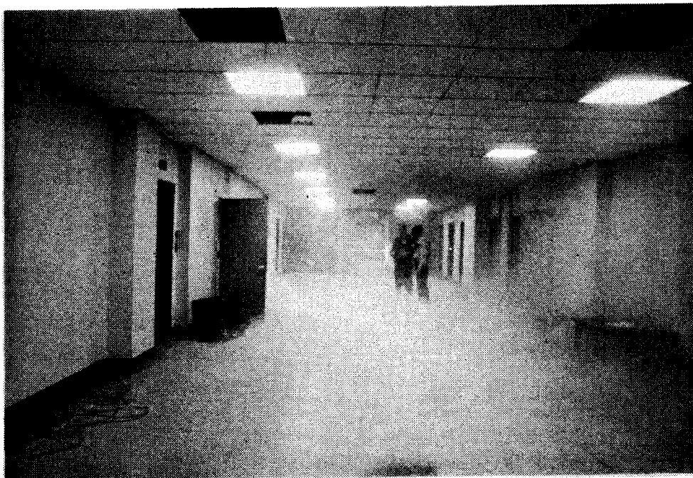
No. 35 - Increasing smoke density in center lobby area. Note open bulkhead door leading from the source of generated smoke.
