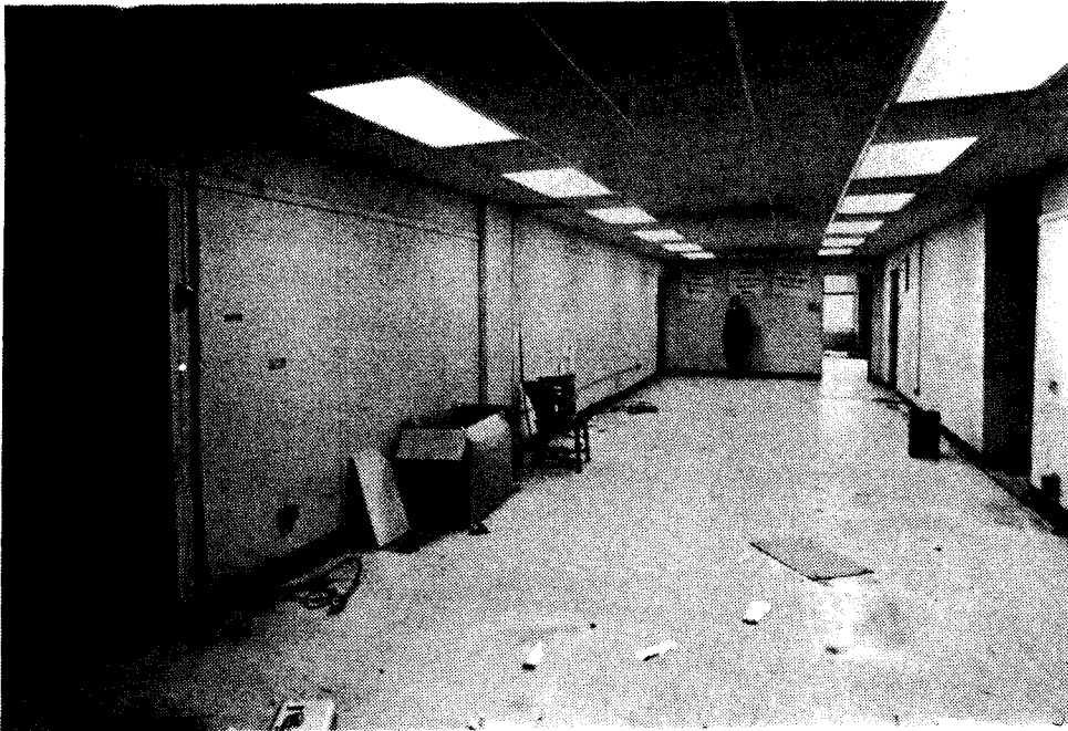
No. 68 - Original site for Fire Test No. 3 can be seen in part through partition opening on the near left. View looking south in 10th floor south end of west wing.
