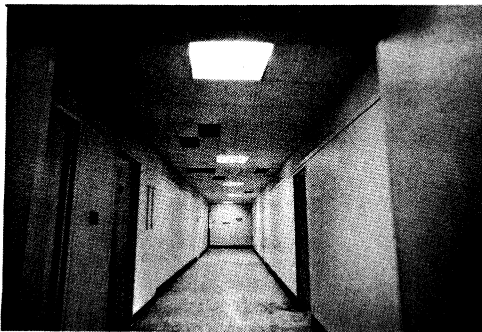
No. 71 - Close-up view of the new site for Fire Test No. 3. Area is behind rear wall of photo in east wing of 10th floor. All ceiling tile replaced before test.
