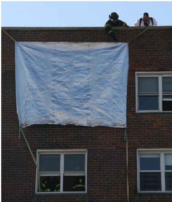
Figure 1.8-5. Wind Control Device Deployed
