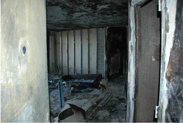
Figure 9.5-43. 5G apartment entrance
