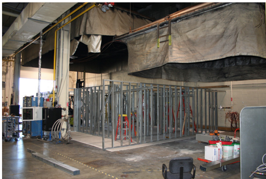
Figure 4.1.1-2. Steel framing for walls of experimental structure inside the NIST Large Fire Facility.
